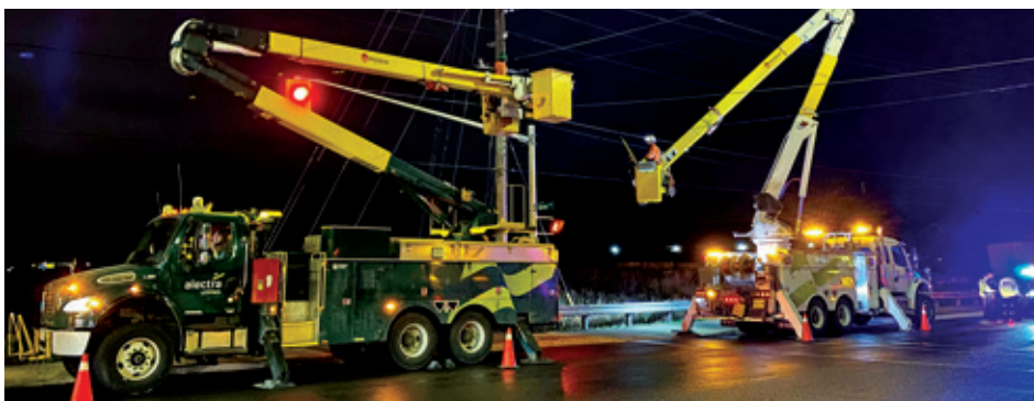
Approximately 20 staff and 12 Alectra vehicles involved to de-energize or lift power lines ahead of the kilometre-long convoy .
