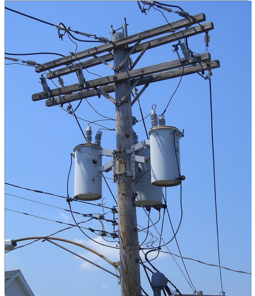
Source: Wikipedia, Distribution Transformer
