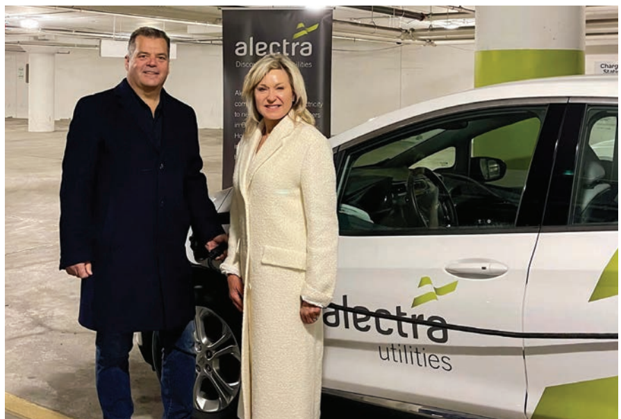
Alectra Inc. President and CEO, Brian Bentz, joined Mississauga Mayor, Bonnie Crombie, to officially announce the installation of 10 Level 2 EV charging stations in the underground parking lot of the Mississauga Central Library.
