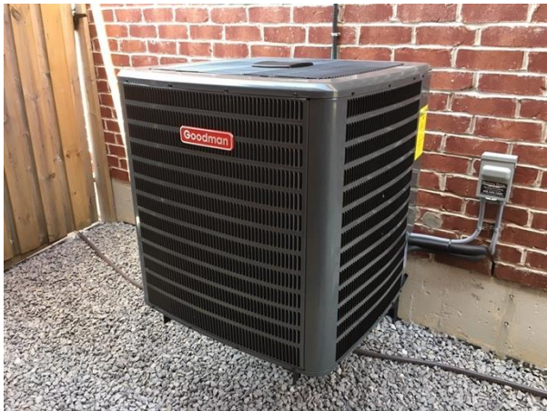
Air-Source Heat Pump
