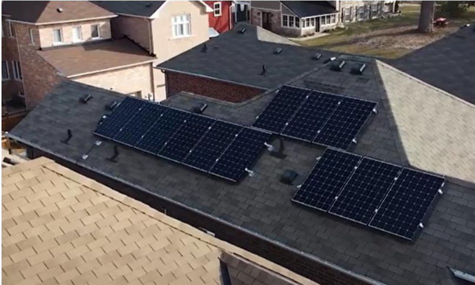
Rooftop Solar PV Panels
