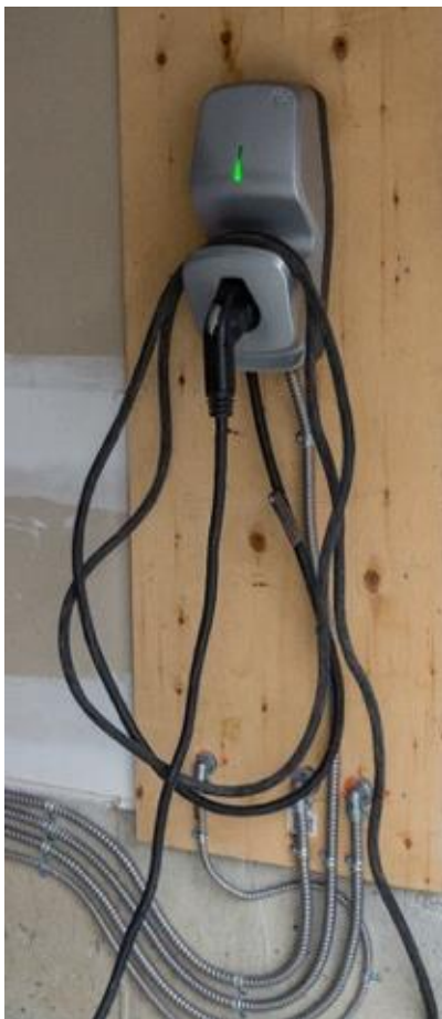
Level II Electric Vehicle Charger
