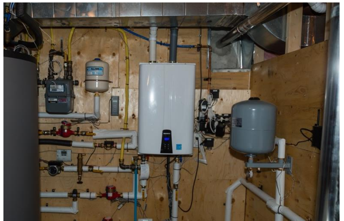
Tankless Water Heater and Piping
